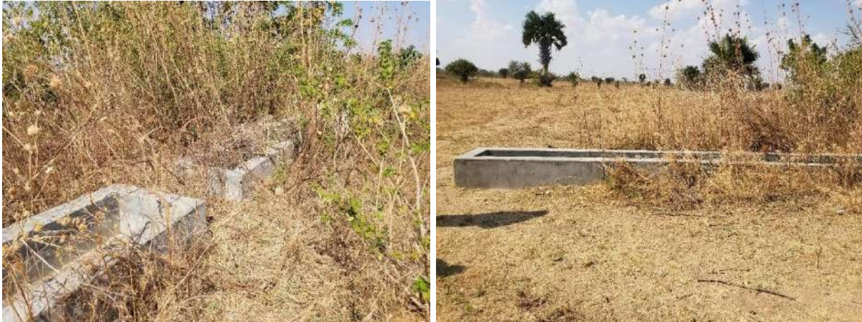
Plate 2-7: Abandoned Livestock watering points at Iboko dam (2024).
